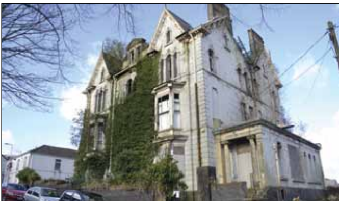
Figure 9: Danbert Hall (Grade II) (At Risk)
